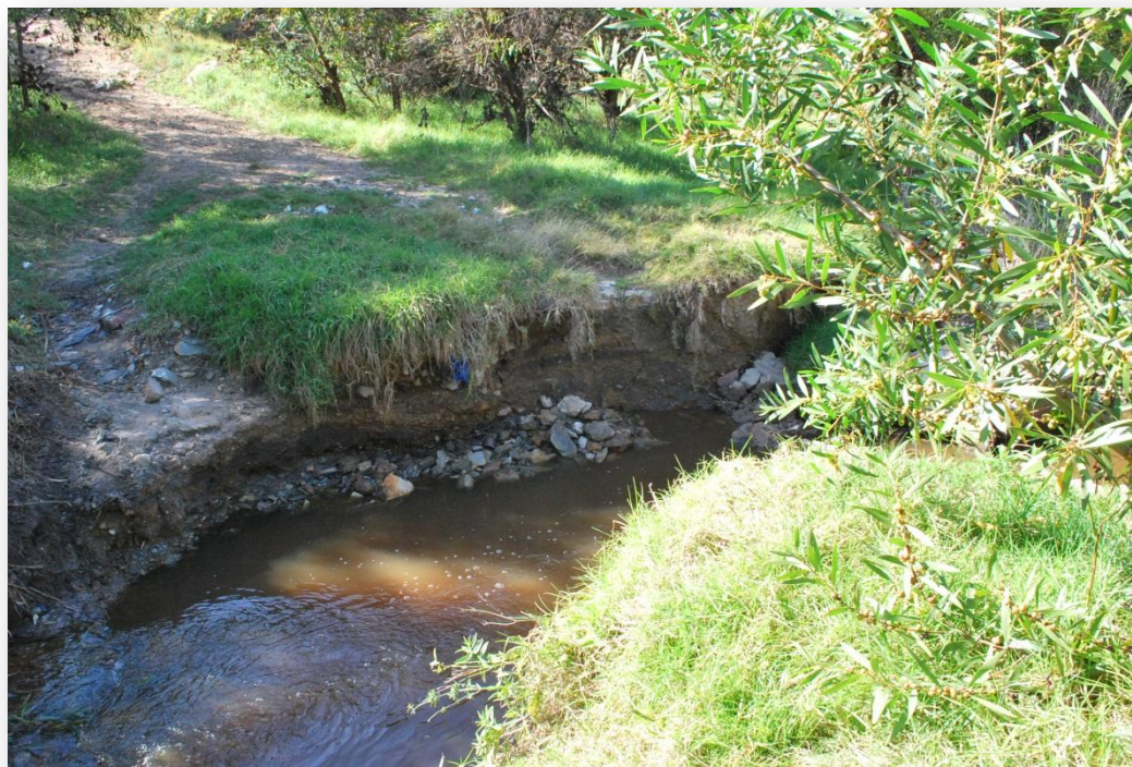
Plate 2: Erosion as a result of an unprotected road crossing and increased runoff velocities downstream of the current water line crossing
