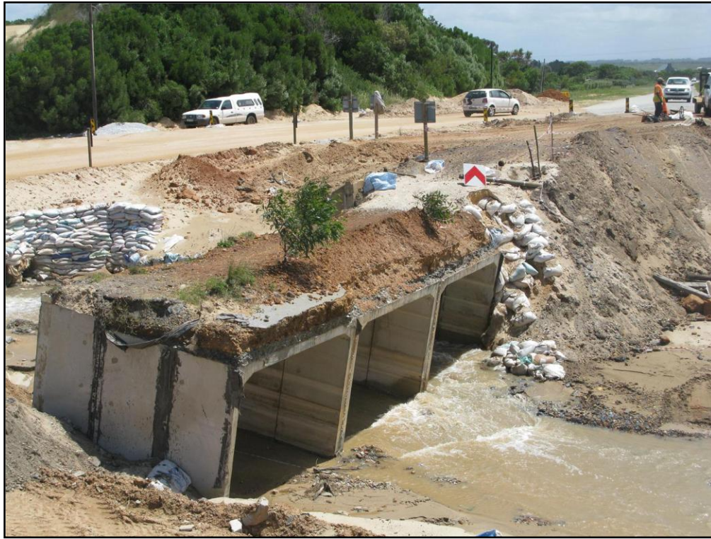
Figure 4: View of the undermined structure that requires replacement.
